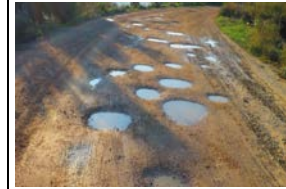
Unsealed road damaged by potholes during wet weather
