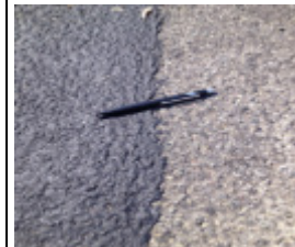
Left side shows condition of 20 yr asphalt surfacing due to binder oxidation
